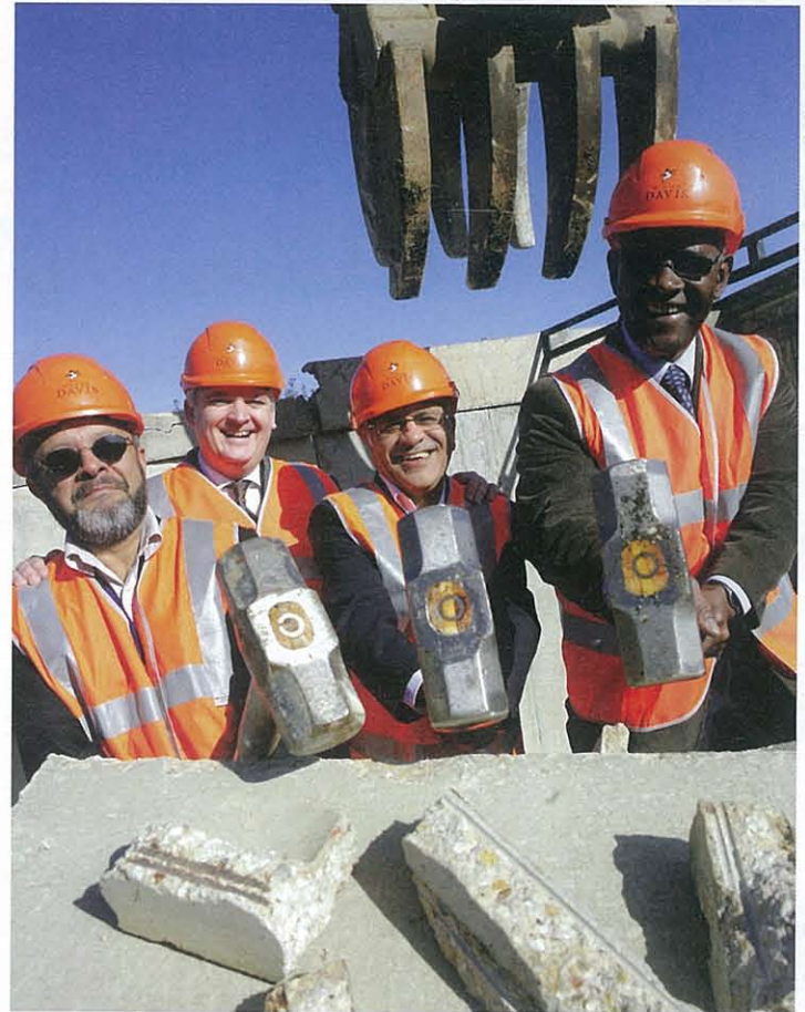
Seven derelict garage sites across Leicester are to be demolished to create affordable family homes. The £5.5m scheme is due to be completed within 12 months, with funding coming from East Midlands Housing (EMH), Leicester Council and the Housing Corporation. Developer William Davis will build 43 homes on the sites, which are overgrown and blighted by flytipping. The properties will be managed by EMH subsidiary, Foundation Housing Association. Pictured (l-r) are Leicester councillor Hanif Aqbany; Chan Kataria, chief executive of East Midlands Housing; William Davis MD Guy Higgins; and Denny Wehner, Foundation Housing Association board member, at the Dillon Way site.
